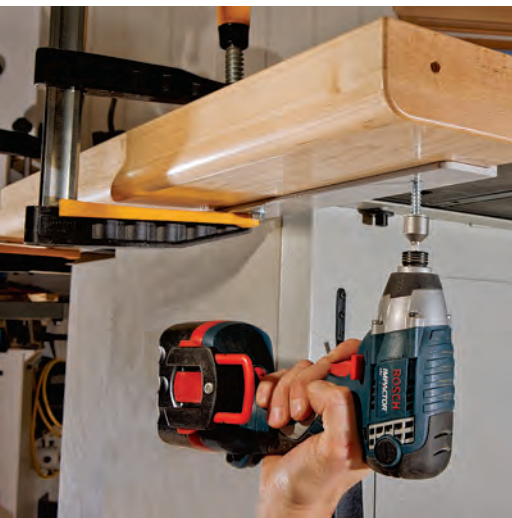
Clamp and then bolt the mounting plate to the saw's fence rail with five 2" lag screws and washers. Keep these fasteners well clear of the miter slots you'll need to rout later.
